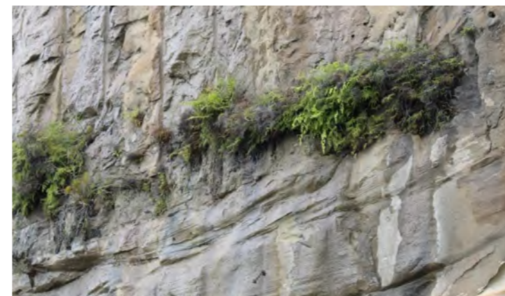
Fig 72. Layers of sandstone on display in the massive cutting of the Eastern Apron. Source: Tyrrell Studio
